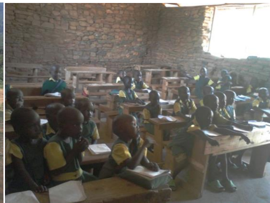
Plate 12: An incomplete classroom
