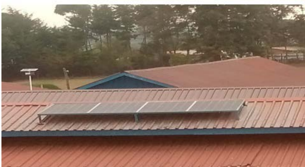
Figure 3.3: Photograph of roof-mounted PV Array at the Institute's Social/ dining hall.
