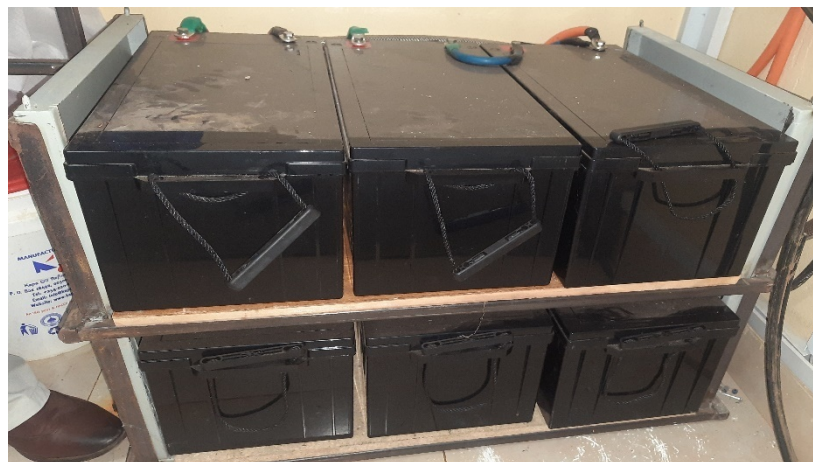
Figure 3.5: Picture of Battery Bank System.
