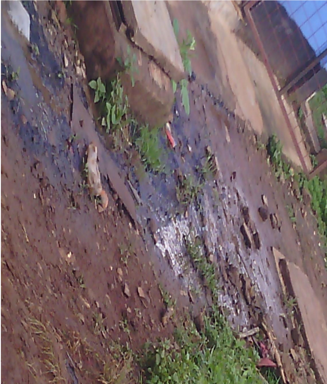
Figure 9: Photo showing poor drainage system
