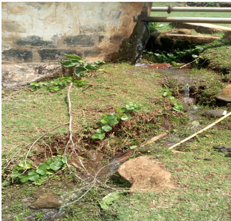
A Leaking Water Tank at Yokot Reservoir
