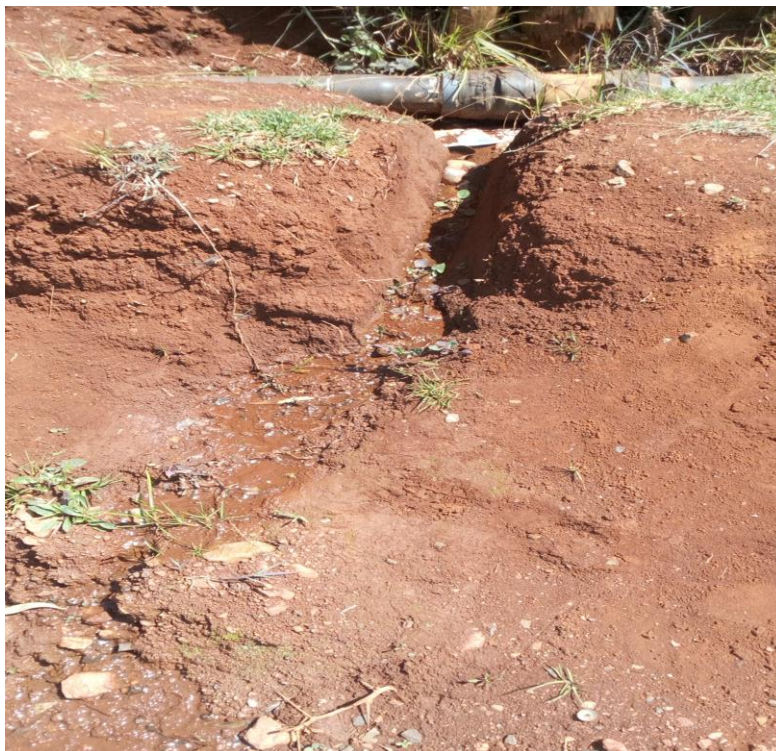
A Leaking Water Pipe at Kapsio Estate
