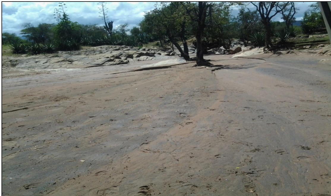
Figure 4.23: Silt deposits on Road camber 500m from Naskuta Primary School. Author (Source 2013).
