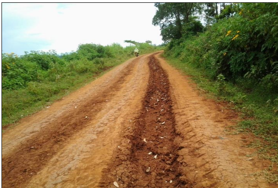
Figure 4.22: Distorted road camber near Kijana Wamalwa Sec School. Author (Source 2013).
