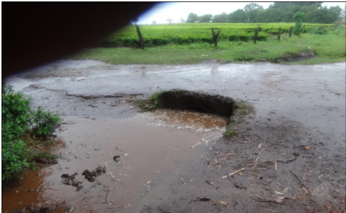
Figure 4.20: Blocked Culvert during Rainy season at Kapchorwa tea factory Junction. Author (Source 2013).
