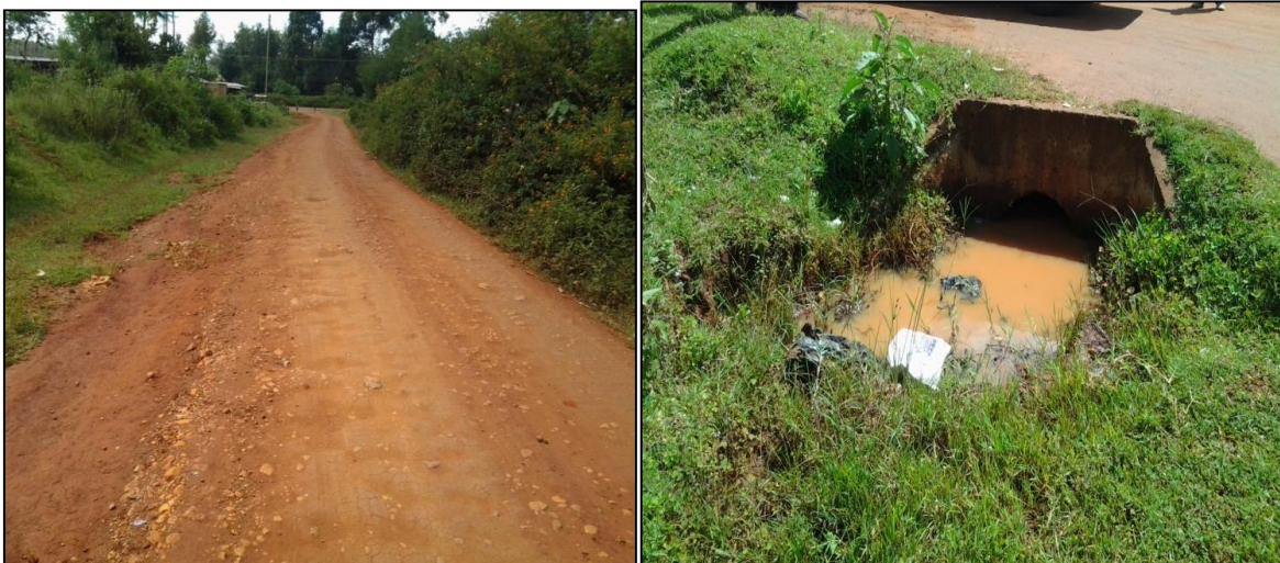
Figure 4.18: Sibanga-Kesegon road at 0+000 km left and right a blocked culvert at Sibanaga-Kitale Junction. Author (Source 2013).
