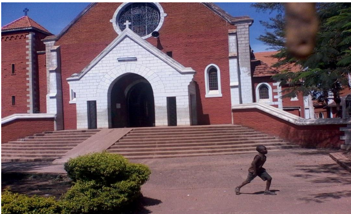
Figure2.1 Main Entrance to a Church in Kisumu City: The ramp superimposed on the stair nosings is too steep to be used by wheelchair bound persons unaided. Source (Author, 2014)
