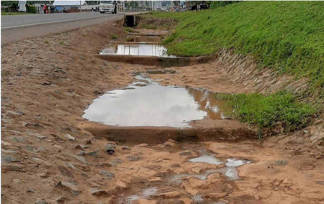
Plate 19: Scour checks on Kakamega-Kisumu road constructed to prevent erosion and slow down the runoff in the trenches.
