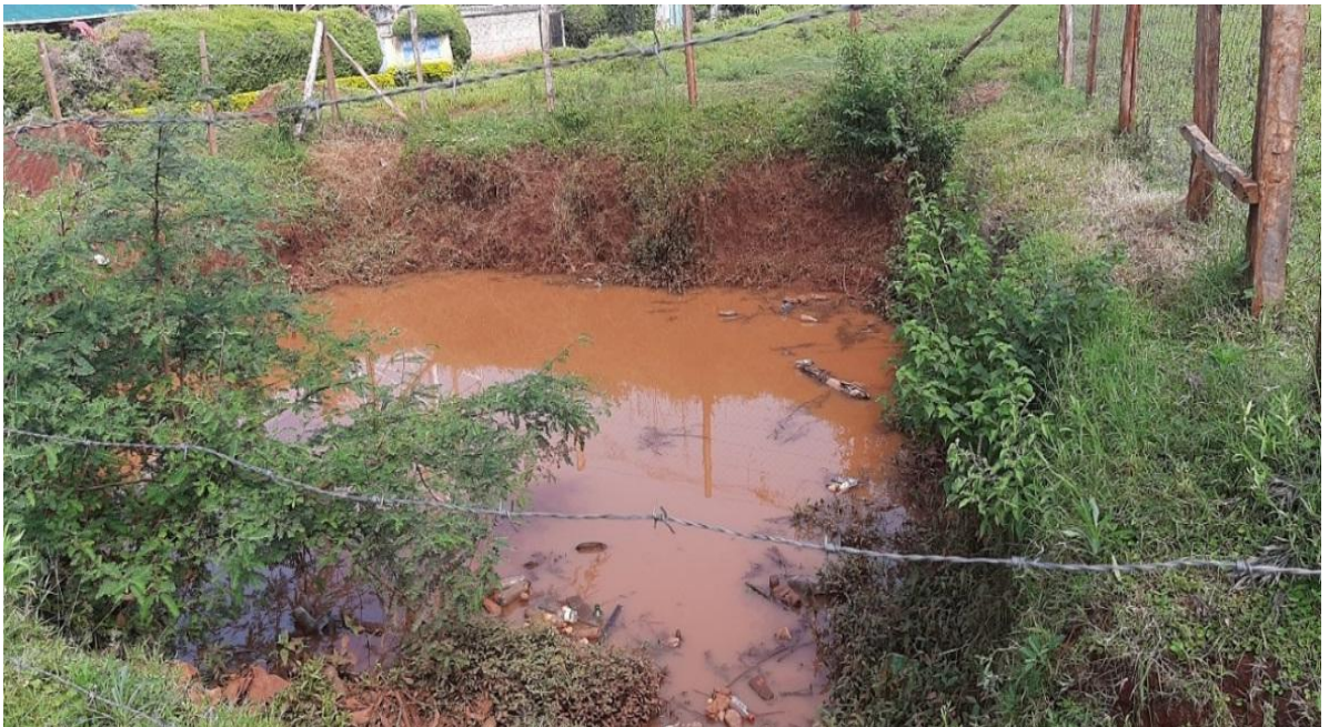
Plate 11: A detention pond near Amalemba Primary to control the flow of runoff from the upper catchment into the informal settlement.
