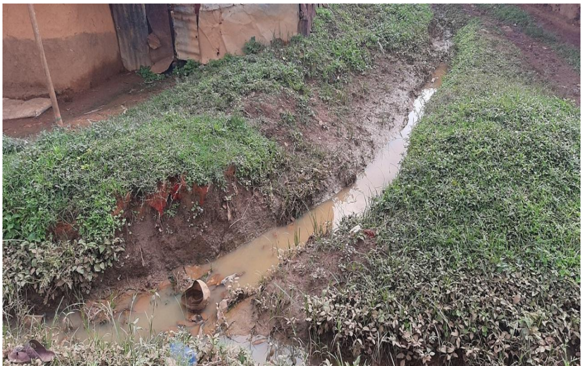
Plate 12: Open drains in Amalemba informal urban settlement as an alternative to enclosed pipe system.
