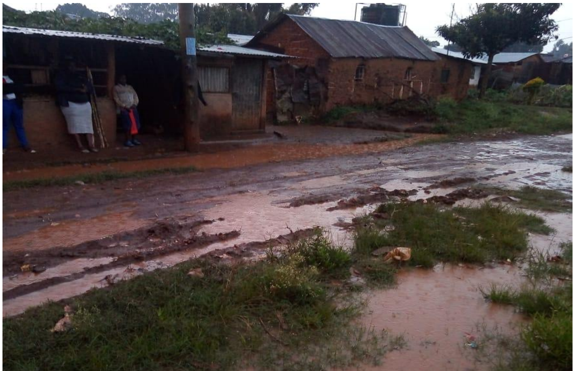
Plate 5: A flooded road in Amalemba informal urban settlement disrupting transportation services.
