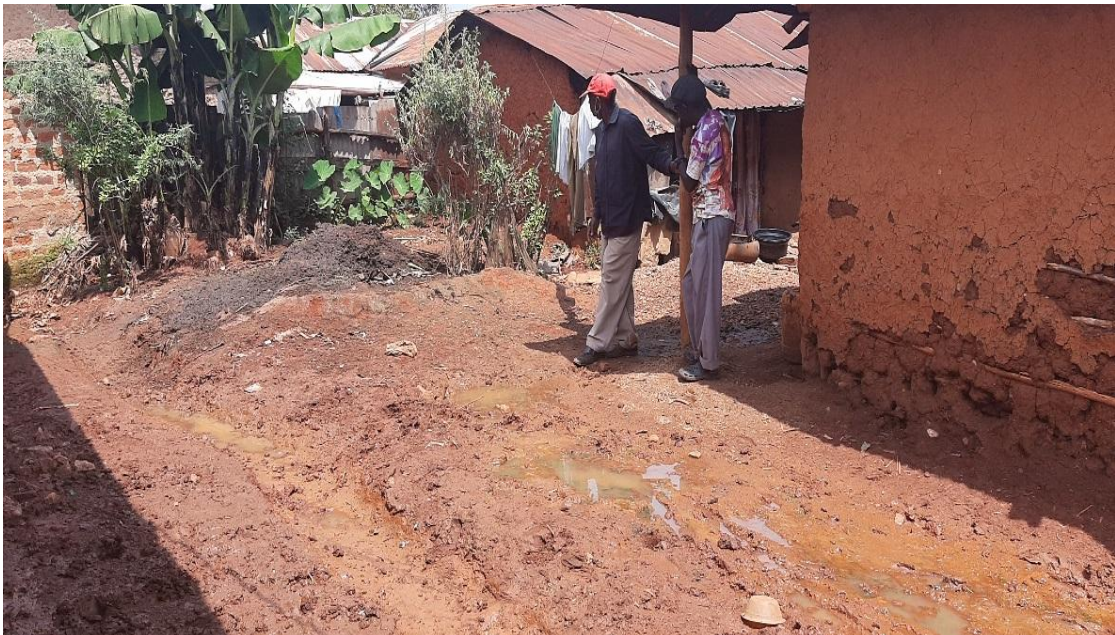
Plate 6: Structural damage to a house in the informal settlement due to flooding.
