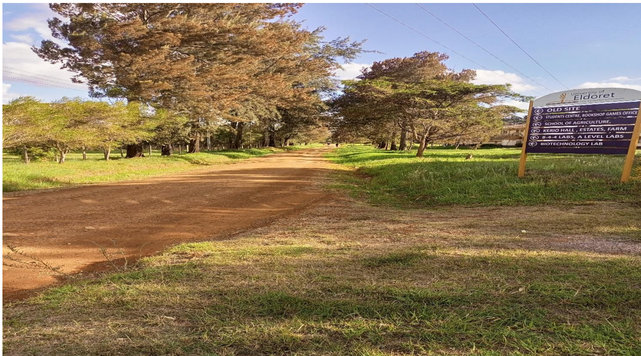
Figure 4. Dispensary-Kerio Hall- Gate B Road link current road condition (April 2023).
